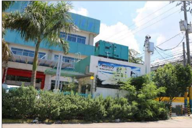
A 125 KVA Powercity generator set placed on a roof deck of a guard house; on standby to provide backup power to a 2-storey building behind. Though this is a flood-free area, it would take a 4.5 meter high of flood before this generator becomes inoperable.
