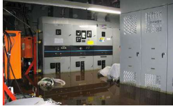
Flooded switchgears of the Fukushima Daiichi Power Plant.
