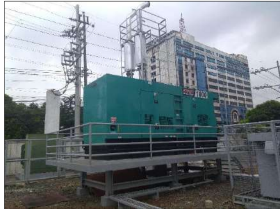
A 1000 KVA Powercity generator set elevated from ground to keep away from at least a meter high flood.
